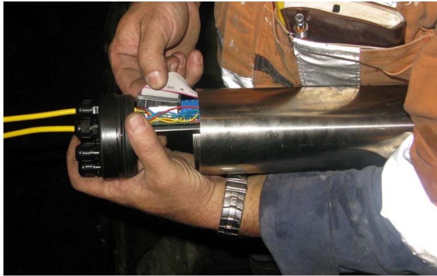
Reconnecting ribbon connector to termination board (RWE termination end cap shown)
